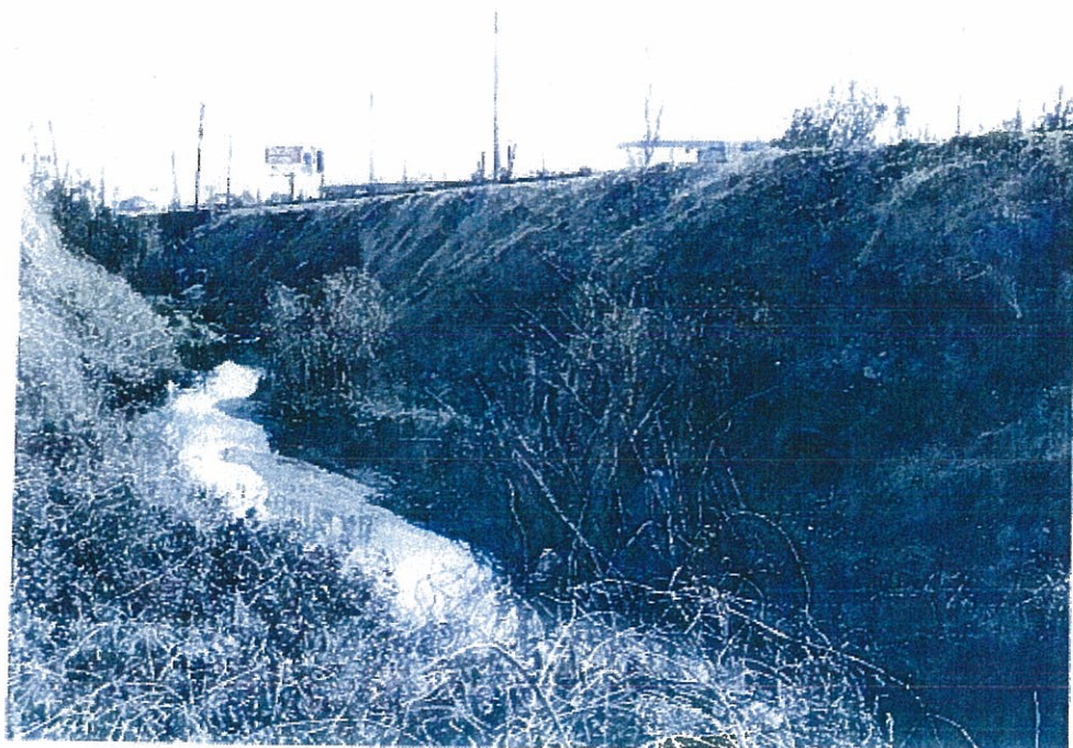
Inlet pipes to railroad ditch
