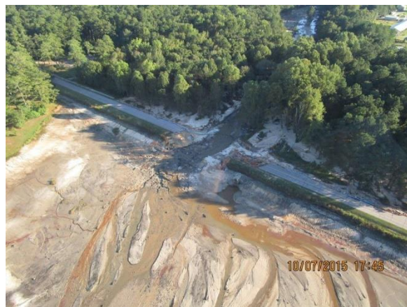
Semmes Lake Dam failure
